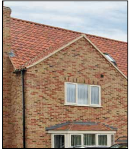
F.52: Mix of coloured brick on new builds. (Photo © AECOM 2022)
